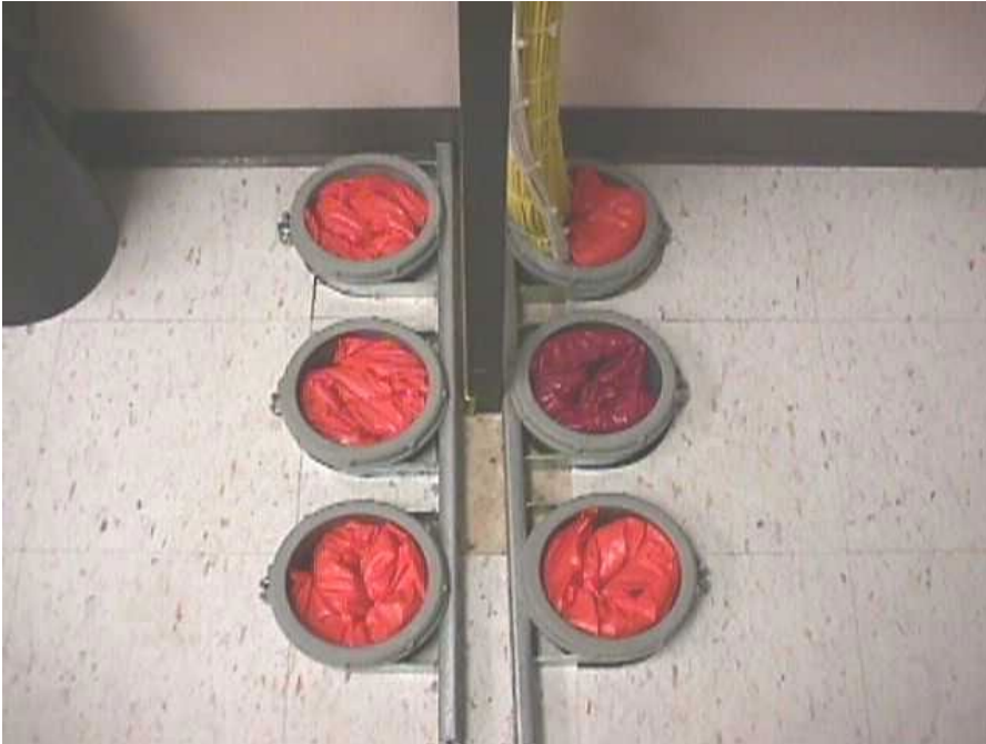
Properly Fire-stopped using SpecSeal™ Intumescent Pillows
